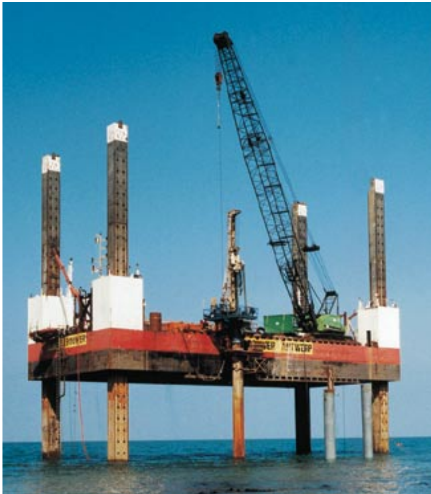
Pile drilling at Lundy Island (Wales) executed by the Zeebouwer, a jack-up owned by the DEME group. This jack-up with a leg length of 42 meters has a payload of 600 tons.
